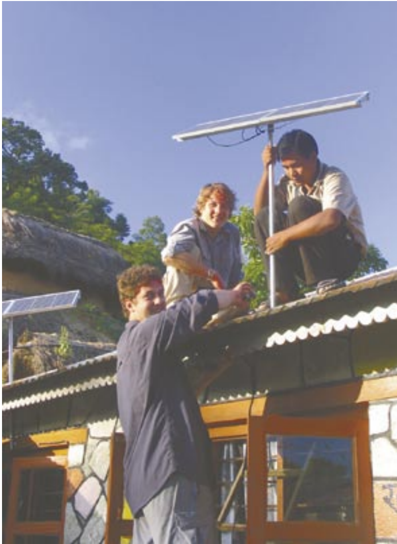
Tane (left) and Harry (centre) are ably assisted by the HLF technician, Mr Ram, installing the first of the five pole-mounted solar panels.
